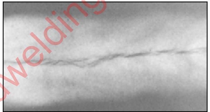
Figure 11: Radiograph Showing Longitudinal Weld Cracking
